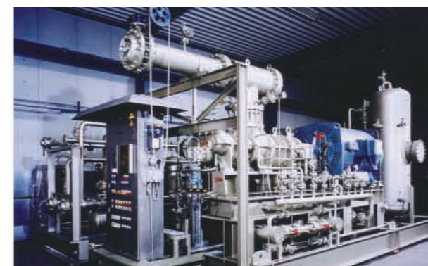
Carbon dioxide gas compressor
