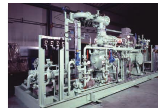
Methyl chloride compressor
